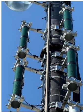
<Base Station with Perovskite Solar Cells>
